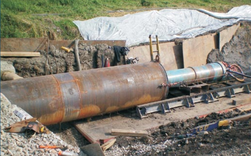
Trenchless pipe installation under Glover Road and CP Rail Tracks for the Township of Langley.
